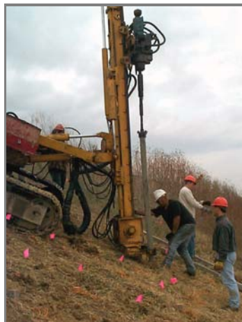
Recycled Plastic Pins are driven into a slope with the percussion hammer from a Davey-Kent Model 100B, track-mounted drilling rig.
