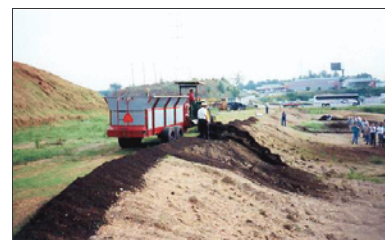
A compost blanket being spread on an unvegetated slope to prevent erosion.
