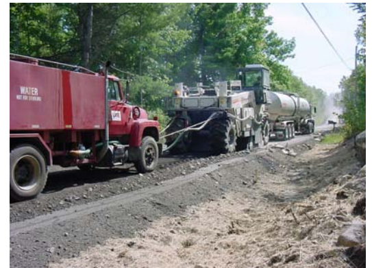
Reclaimer pushing the asphalt tanker and introducing the foamed asphalt into the base. Water truck is towed by reclaimer. Water is introduced at foam spraybar, and aids compaction of the base.
